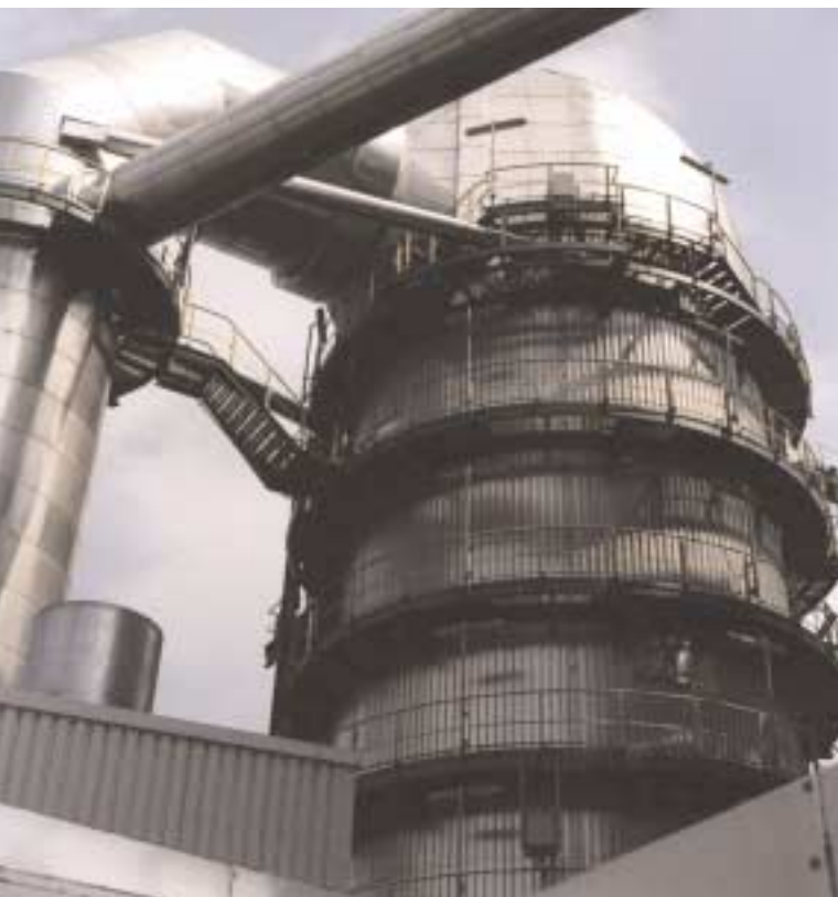
Flue Gas Desulfurization Unit “Chemische Werke Hüls, Germany” (Source: Krupp, Thyssen Nirosta)
