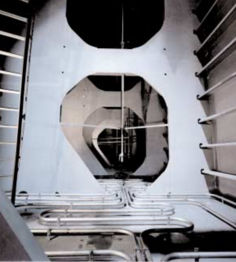
Inside a 2205 (1.4462) Tank on a Marine Chemical Tanker (Source: Krupp Thyssen Nirosta)
