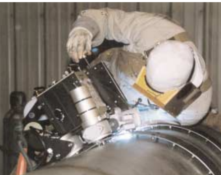
Mechanized Welding of Large Diameter Duplex Stainless Steel Pipeline on Alaska's North Slope (Source: Arco Exploration and Production Technology)
