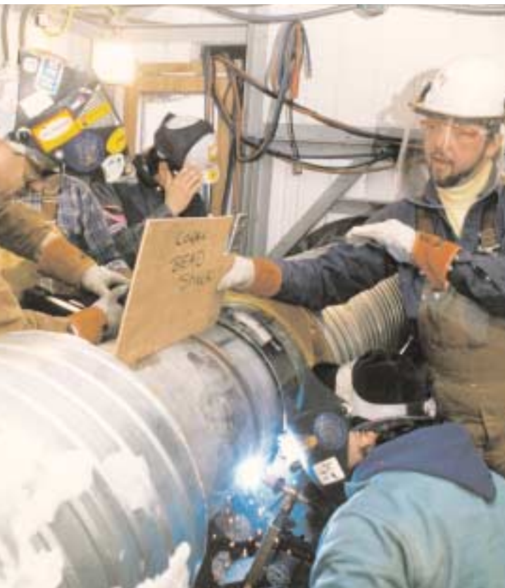
Mechanized Welding of Large Diameters Duplex Stainless Steel Inside Welding Shack on Cross-Country Pipeline (Source: Arco Exploration and Production Technology)
